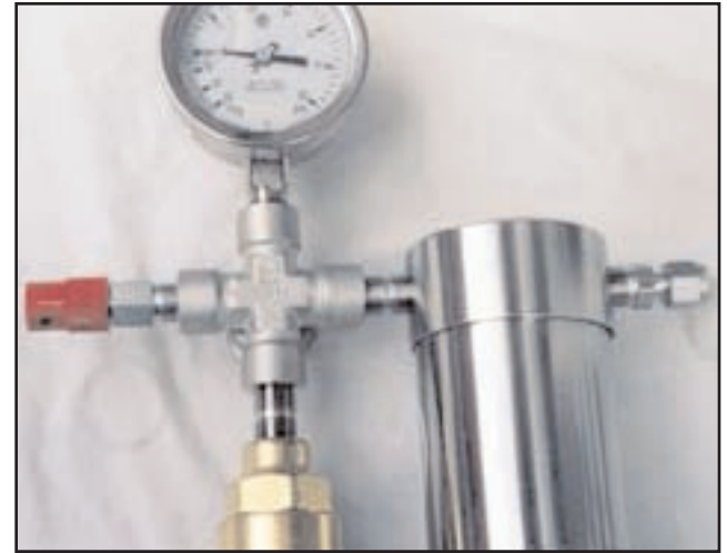
The relief checkvalve, pressure/vacuum gauge, and tops of a flash-back arrestor and coalescer.
